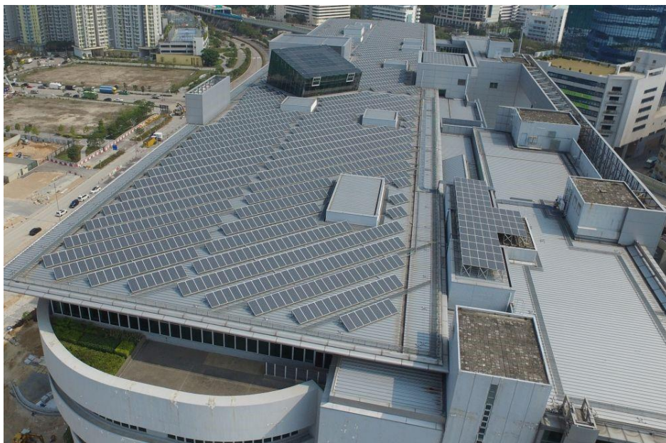
Figuur 87 Origineel PV Roof systeem EMSD headquarters, Hong Kong. Bron: foe.org.hk
